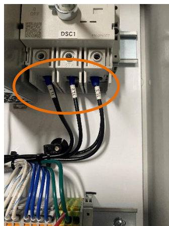
Figure 13: Output Terminal Connections on the Main Disconnect Wired for Three-Phase.
